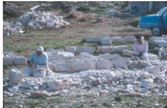
Figure 10: Stonecutters preparing specific stones for a building (Van and Anita Parunak, Apr 1975)
